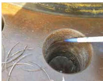
▲ A typical thread before refurbishment.
